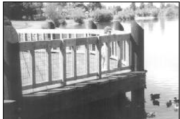
Treated wood piers allow the public closer access to the water than ever before.
