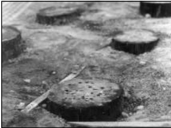
Project with salvaged piling. Note the extensive marine borer damage that resulted in "red tagging" and significant expense to the contractor.
