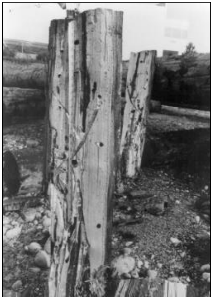
Appearing sound, this salvaged piling disintegrated when driving, exposing extensive rot and marine borer damage.
