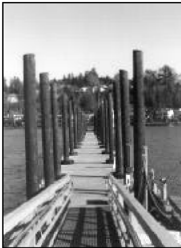
Treated wood is an important product for the construction of marinas and personal use docks.
