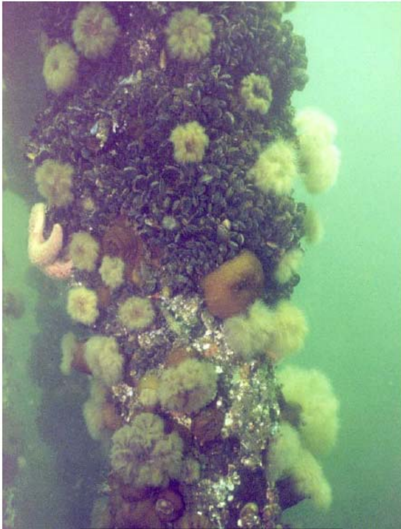
Sooke Basin Creosote Treated Piling After 4 Years In Place
