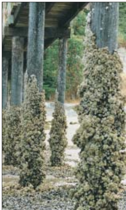
The personal use pier shown here is constructed of creosote-treated piling with ACZA-treated walkways
